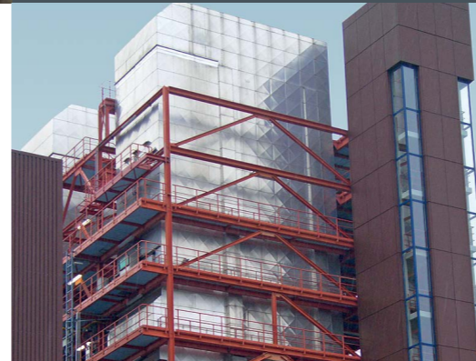
Proven use in waste incineration plants
