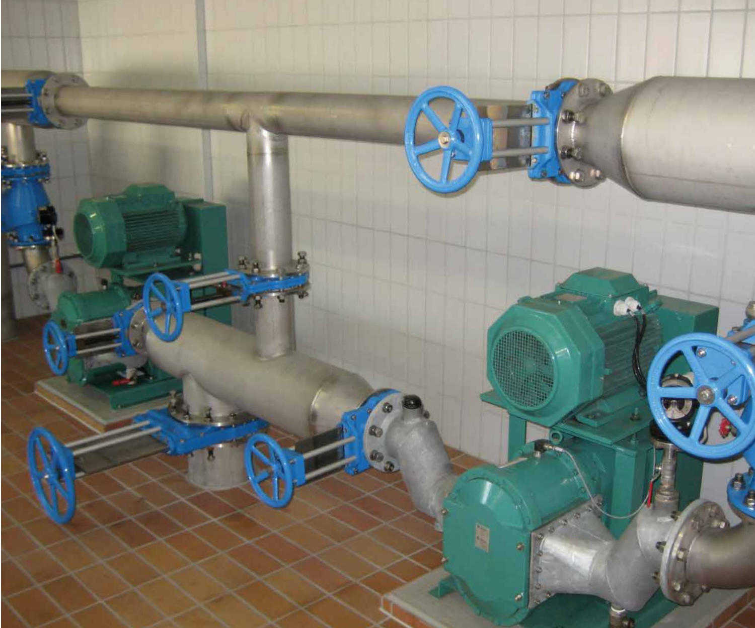
TORNADO® rotary lobe pumps in digested sludge recirculation
