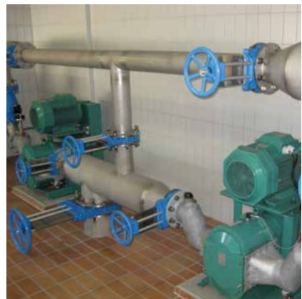
TORNADO® rotary lobe pump conveys digested sludge in the sewage plant
