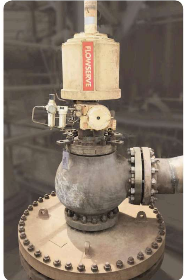
Valtek Survivor valve installed in flashing slurry letdown service
